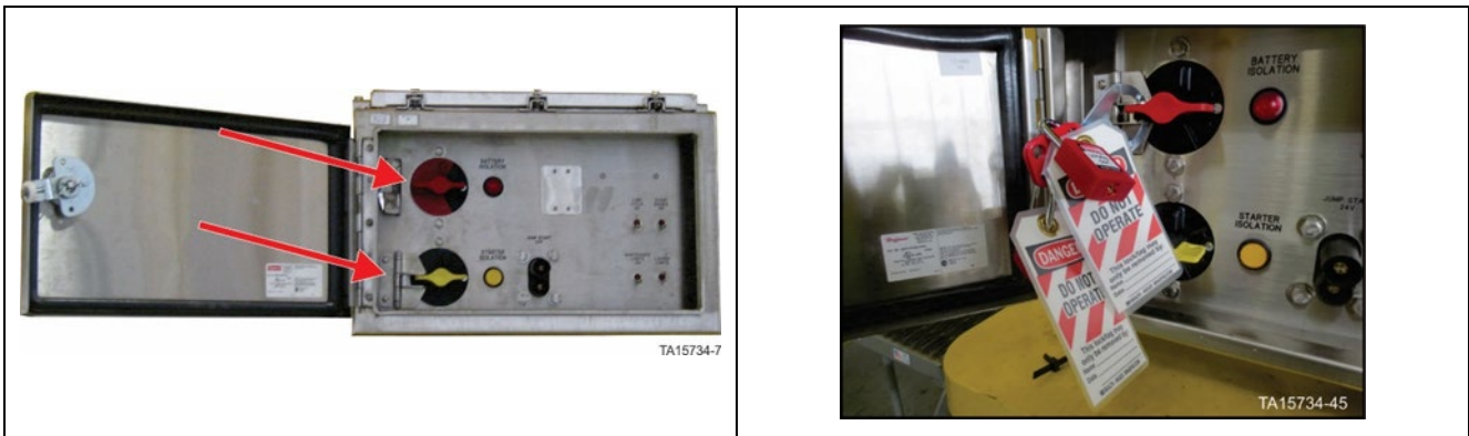
Figure 5. Battery Isolation Box – Battery isolation switch in OFF position with locks in place
