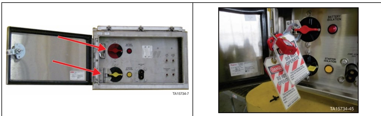
Figure 23. Battery Isolation Box – Battery isolation switch in OFF position with locks in place
