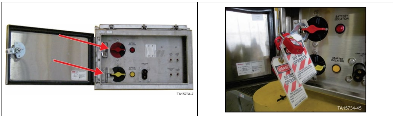
Figure 31. Battery Isolation Box – Battery isolation switch in OFF position with locks in place
